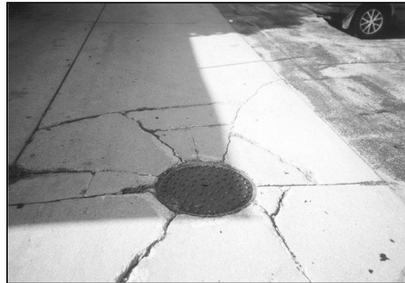
Cracked pavement in need of repair.
