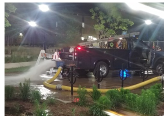
Hydrant Flushing Insuring the integrity of the water system and providing high quality water
